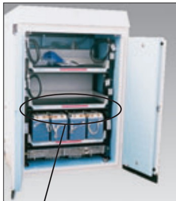
Pull-out drawers for easy maintenance of batteries
