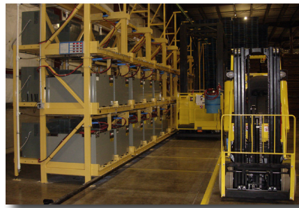
Forklift Battery Station
